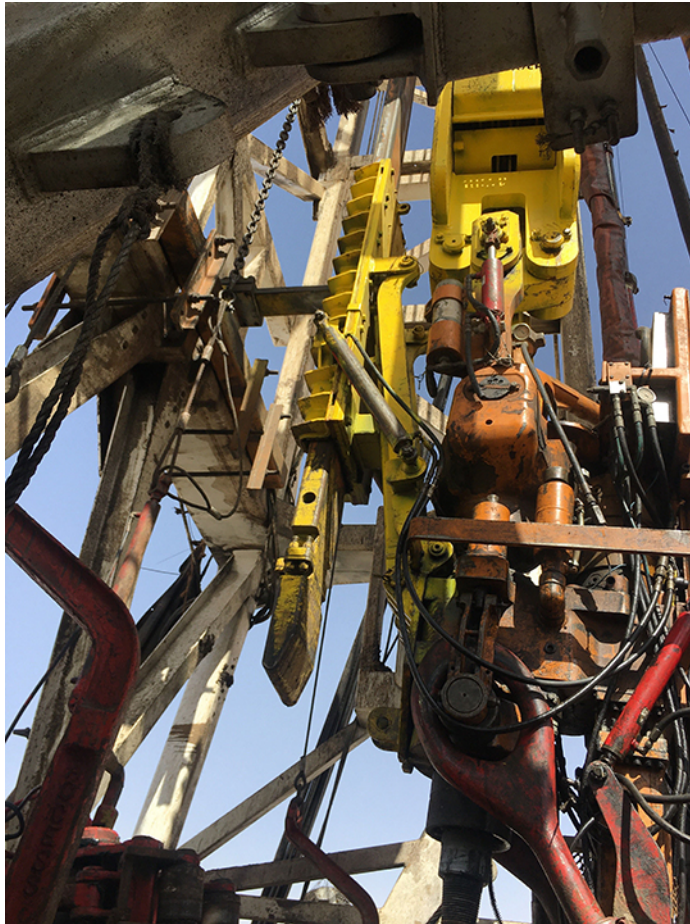
Figure 1: Noticeable Tilt of HMI Top Drive
